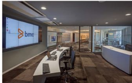
The Network Operating Centre on Level 10.
